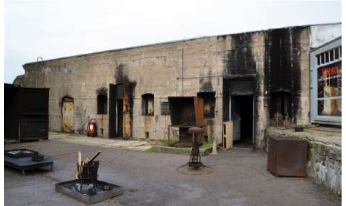
Fig. 10: Traces of fire in the self-protection training area of the fort near Marken-Binnen
